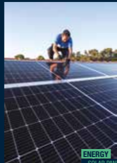
ENERGY - SOLAR PANELS
