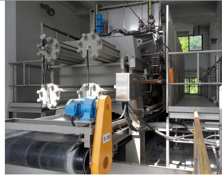
Rear view of the new sludge dehydrator facility at the Ulsan site.
