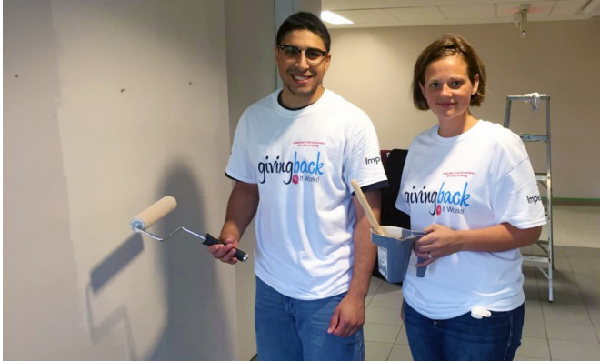
Helal Elkolaly, Operations Engineer, and Erin Dasilva, Associate Project Controls, painting the corridor of the Huron House.
