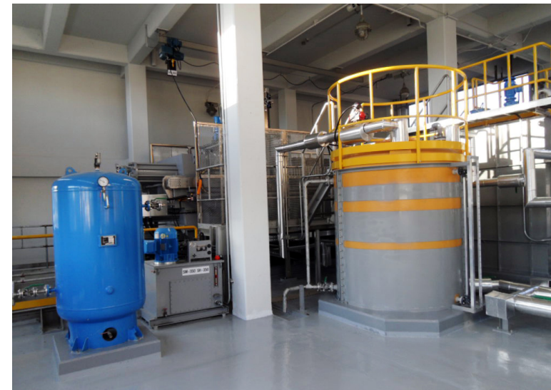
Supplementary facilities of the mechanical dehydrator to dewater the sludge.
