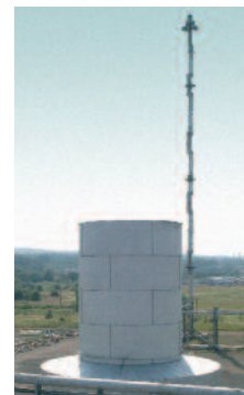
Ground flare and high level flare
