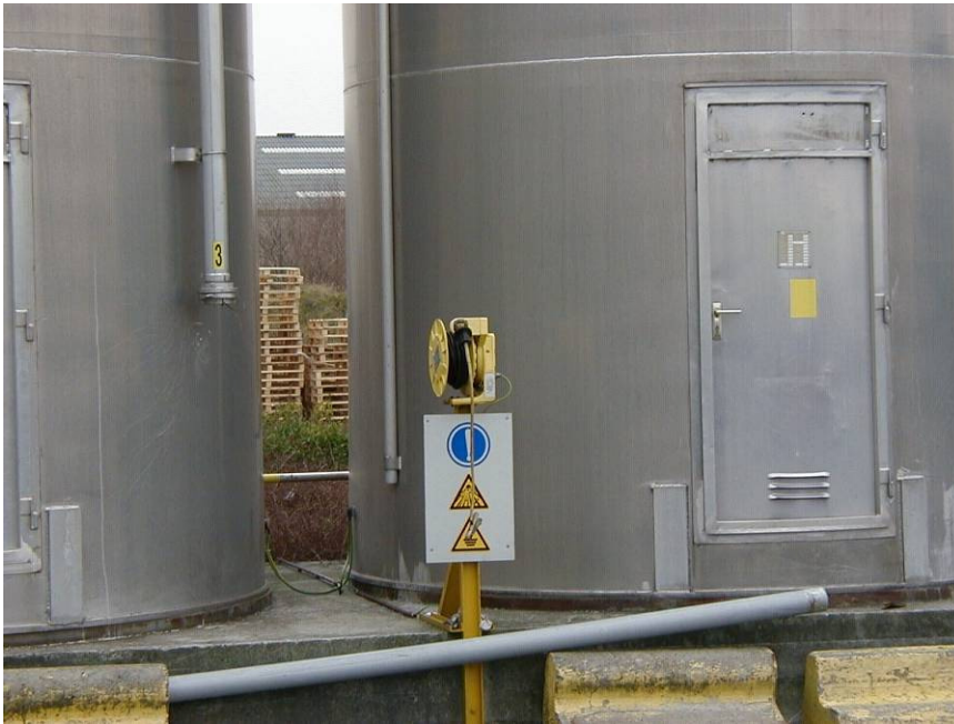
Earthing cable and earthing pictogram
